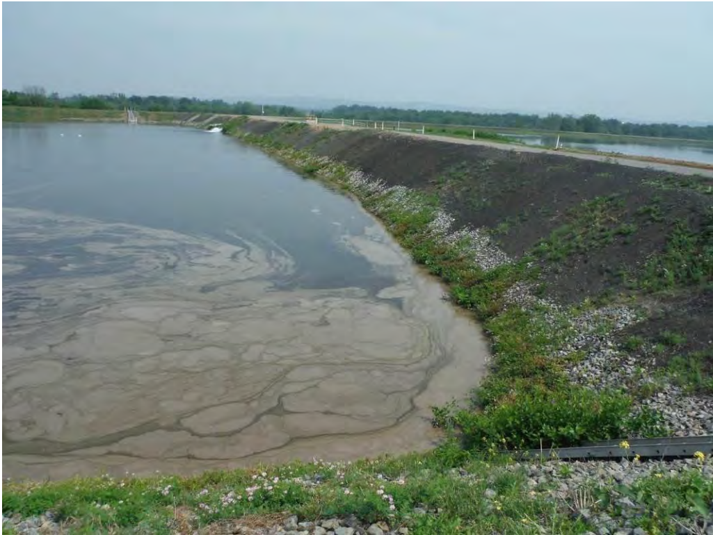
Photo 36 – The downstream face (C side) of splitter dike between Sub-basins B and C.
