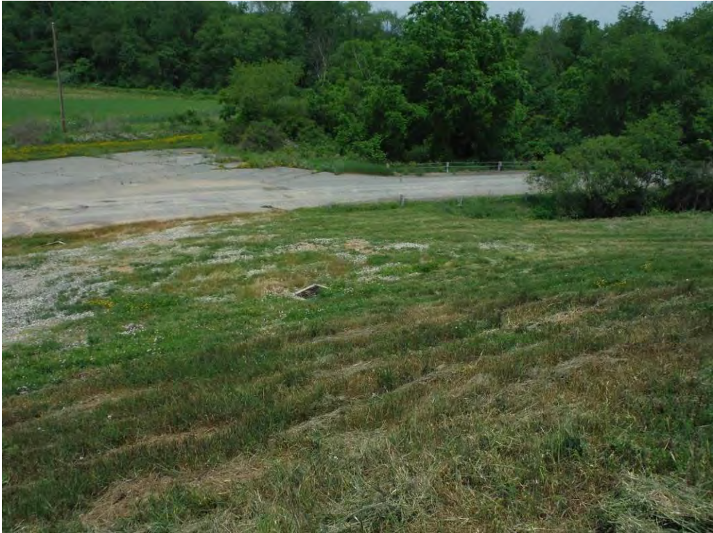
Photo 24 – Alignment of the drain line at the east end of the north embankment. The two lower catch basins can be seen. Both catch basins had seepage entering the basin from improperly sealed penetrations, with surface subsidence above.
