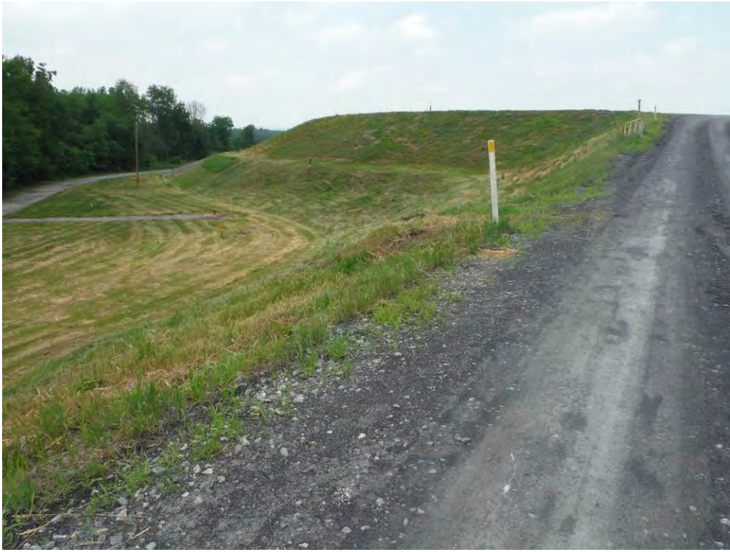
Photo 28 – The downstream slope of the northwest embankment, looking northeast from access road.
