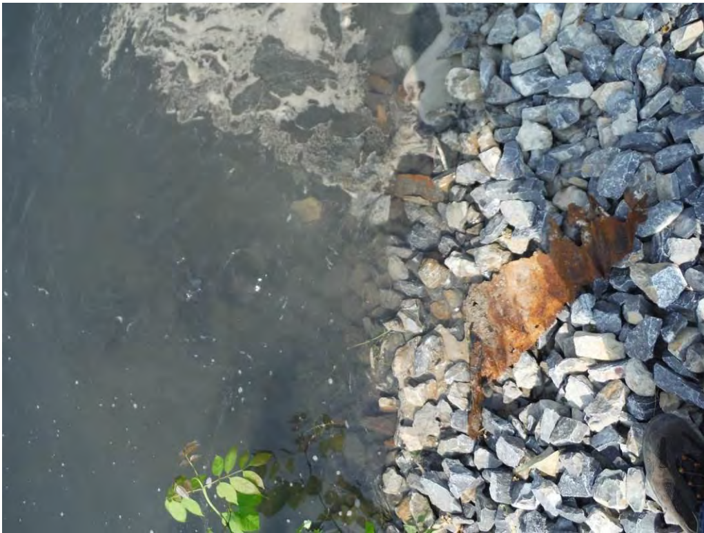
Photo 38 – Abandoned, corroded CMPs in the splitter dike. –Boil observed at outlet of one abandoned pipe.
