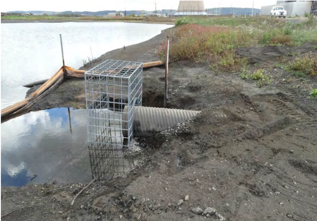
Photo 37a – Trash rack installed at upstream end of intake between sub-basin B and C
