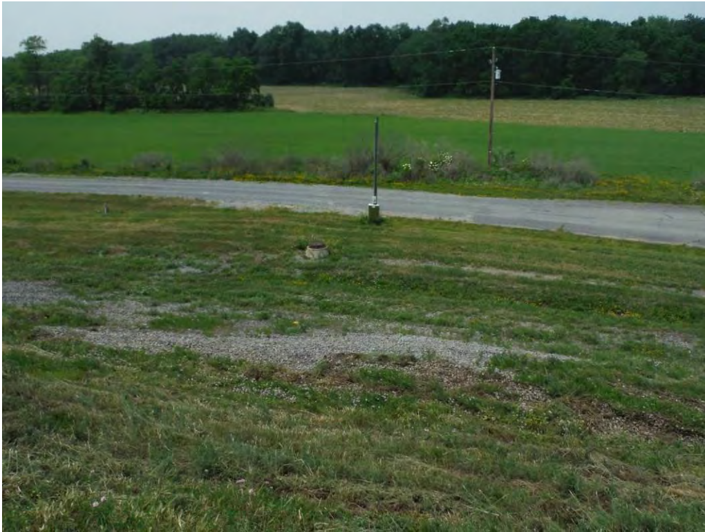
Photo 25 – East end of north embankment, showing gravel stabilization berm and the manhole that houses dewatering well 4. Wet areas have previously been observed here, and were damp during the 2015 inspection.
