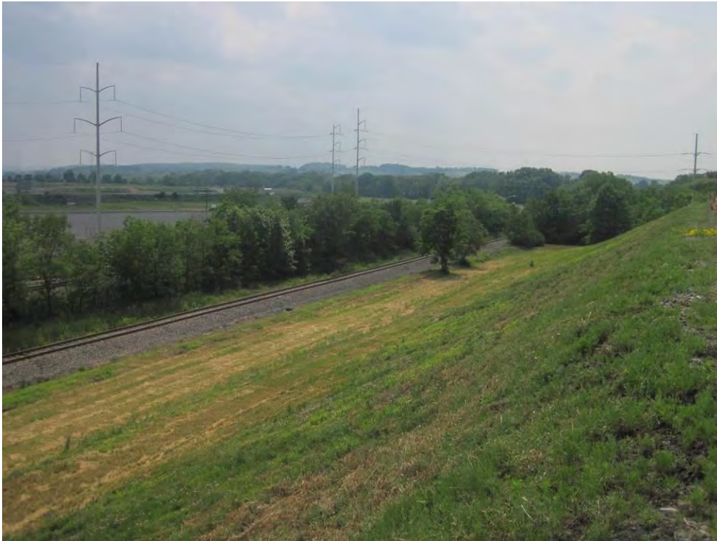
Photo 14 – Downstream slope of southwest embankment, looking northwest from near the splitter dike between Sub-basins B and C.
