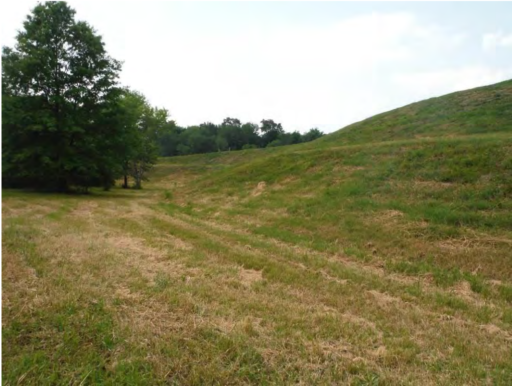
Photo 13 – North end of southwest embankment and access ramp. Wet areas observed in previous inspections along toe were observed dry or damp in 2015.
