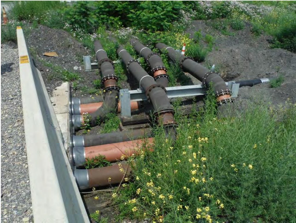
Photo 33 – Cribbing at discharge pipe bend near bridge abutment, which was modified in 2014.
