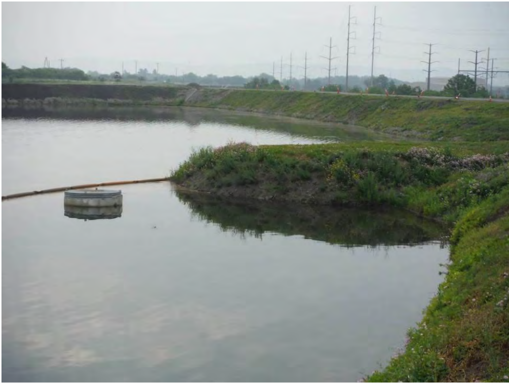
Photo 2 – Upstream slope of Sub-basin C looking southeast, showing outlet riser and riprap slope stabilization.
