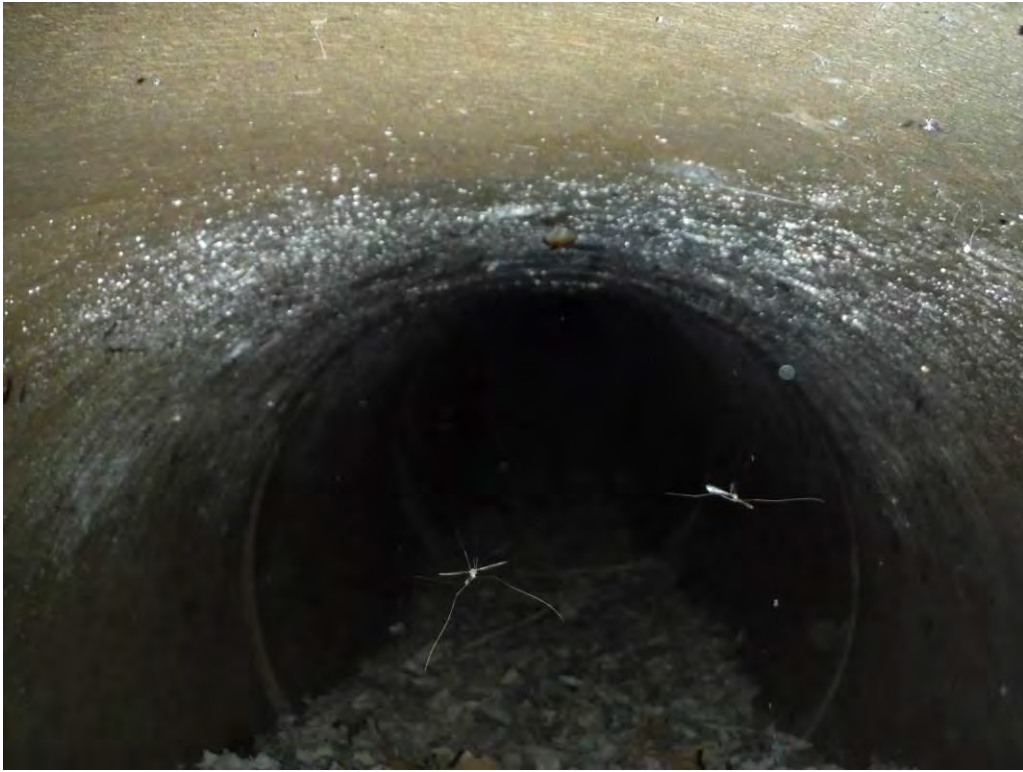
Photo 42 – The outlet pipe of an abandoned outlet structure running from Sub-basin C to Chillisquaque Creek. View inside the RCCP outlet pipe.
