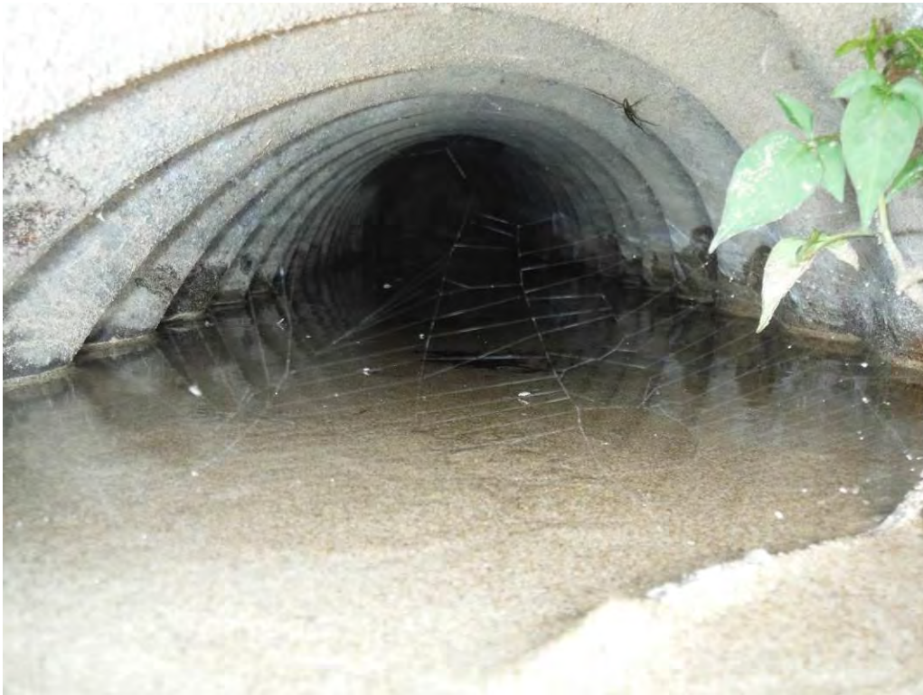
Photo 4 – View of the interior of the 12-inch CMP at the waterline at upstream slope of Sub-basin C, showing pipe partially submerged. A photo of the pipe interior taken in 2014 showed the pipe partially clogged.
