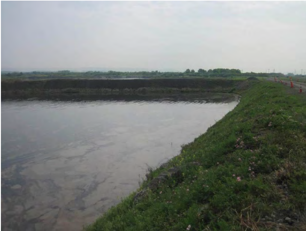
Photo 3 – Upstream slope of Sub-basin C looking southeast. The 12-inch CMP at the waterline was half submerged during the 2015 inspection. There was no current or other evidence of flow entering the pipe. The purpose of the pipe and the alignment of the pipe within the embankment is unknown.
