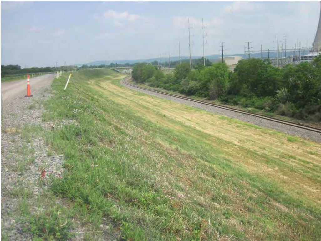
Photo 16 – Downstream slope of southwest embankment, looking southeast from near the splitter dike between Sub-basins B and C. The pipe bridge can be seen in the distance.
