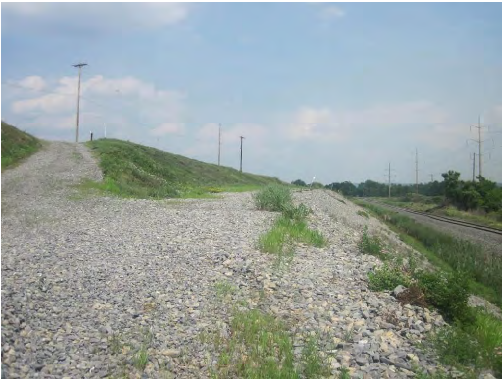
Photo 18 – Downstream slope of the southwest embankment, looking southeast from the pipe bridge.
