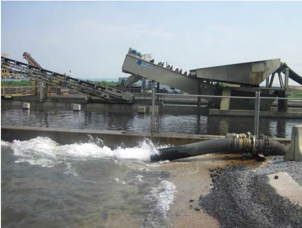
Photo 34 – Ash discharge area, showing the settling basins.
