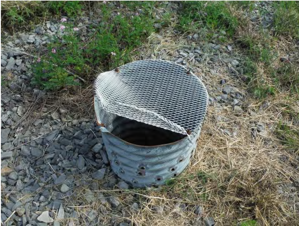
Photo 29 – The ditch near the west end of the north embankment, adjacent to dewatering Well No. 1. Note the damaged screen on the top. The ditch was drier than previous years.
