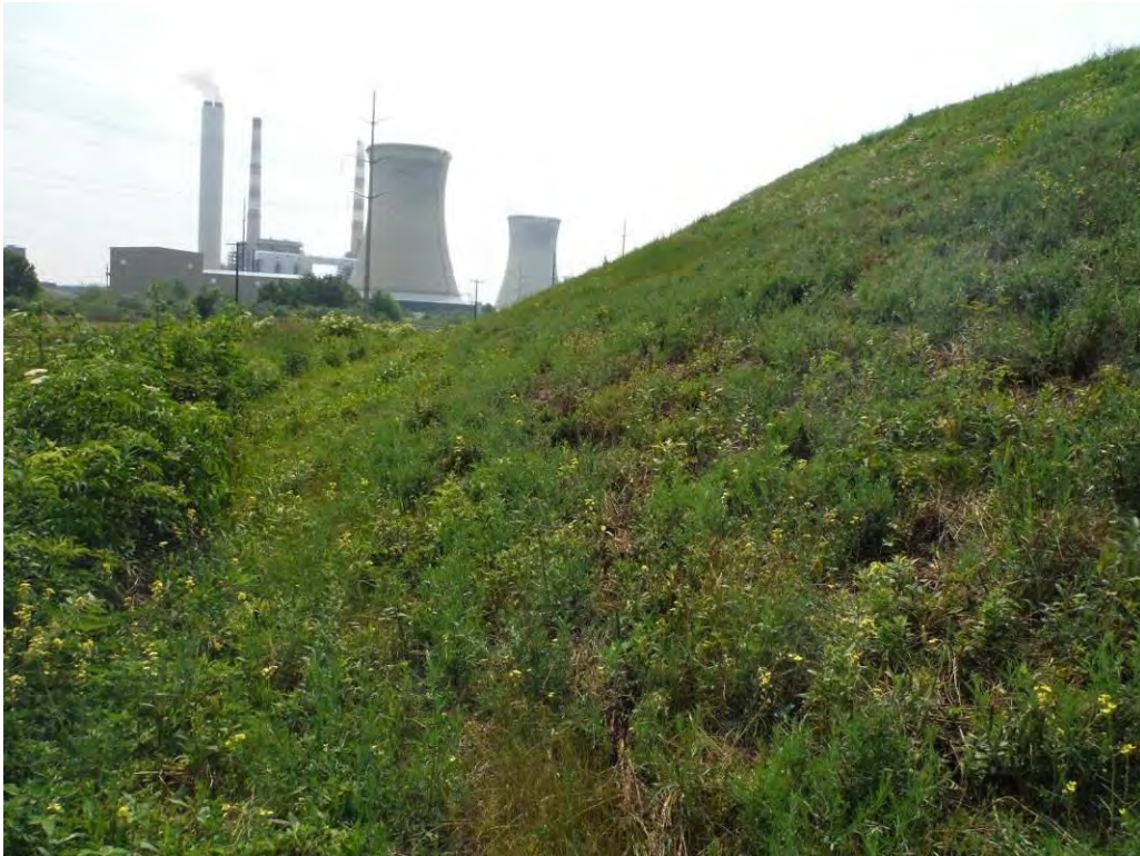
Photo 20 – Downstream slope of the southwest embankment, looking northwest from the southwest corner of Sub-basin A.–Note the vegetation overgrowing the embankment toe.
