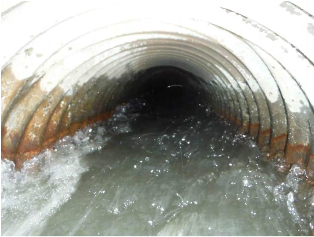
Photo 40 – Splitter dike discharge pipes exhibited signs of corrosion, view of the pipe interior from downstream end.
