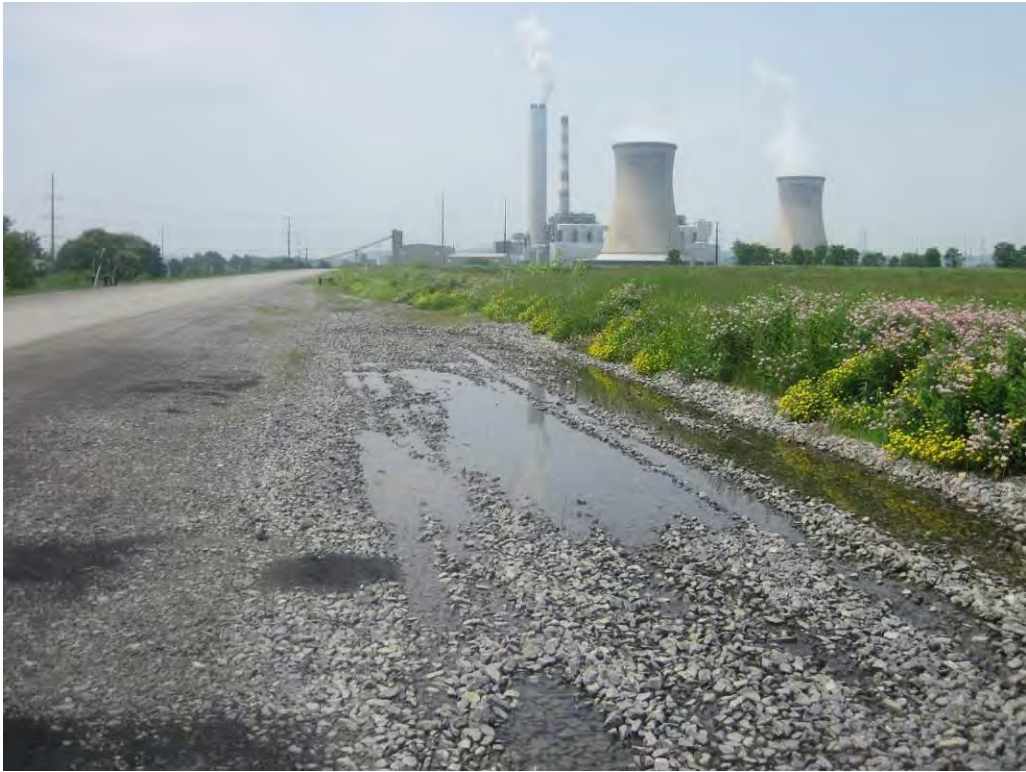
Photo 12 – The closed portion of Sub-basin A at the southeast corner of the ash basin. Note some minor surface runoff ponds along the Sub-basin A dike on the crest road. The crest access road has been regraded to slope toward Sub-basin A, and a drainage swale has been constructed in Sub-basin A dike to drain runoff from the crest access road.
