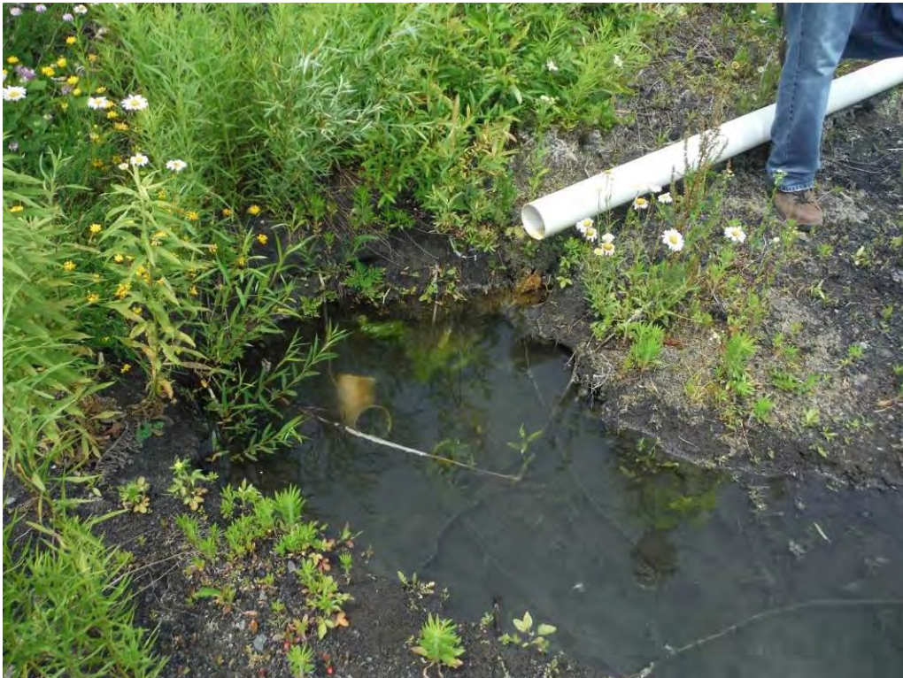
Photo 8 – PVC elbow disconnected from the 4-inch PVC discharge pipe from dewatering well 4, located on the upstream slope of Sub-basin B. Talen reported that a modified swale now conveys this discharge.
