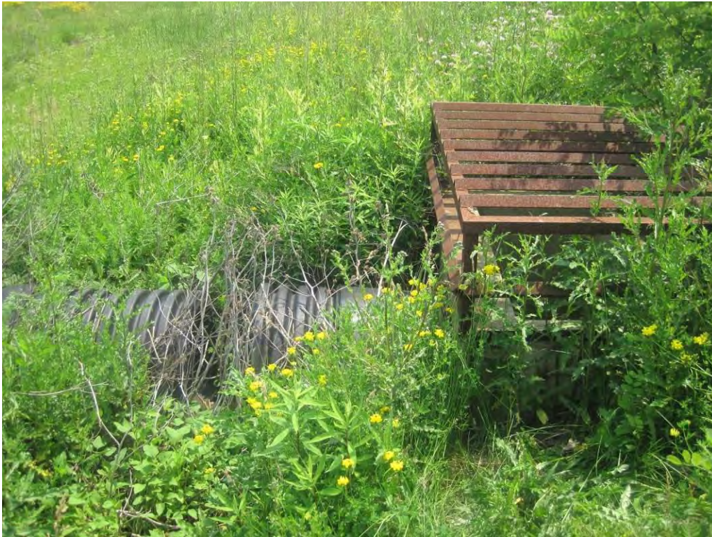
Photo 10 - Cut out in the catch basin drainage pipe in Sub-basin A that has the potential to fill with mud or debris. Talen noted that the pipes were capped subsequent to the inspection.
