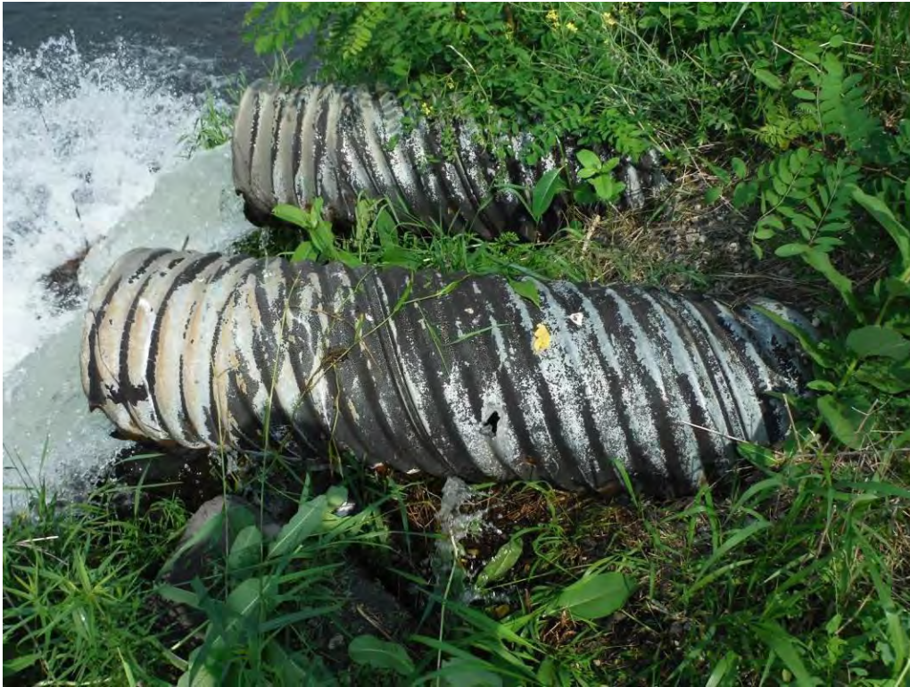
Photo 39 – Active splitter dike discharge pipes exhibited signs of corrosion.
