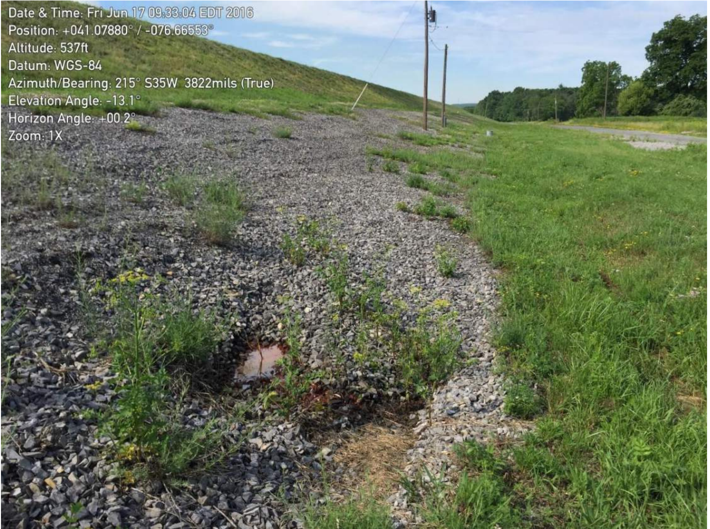
Photograph 3 – Seep at Toe of Northern Dike Slope (looking west)
