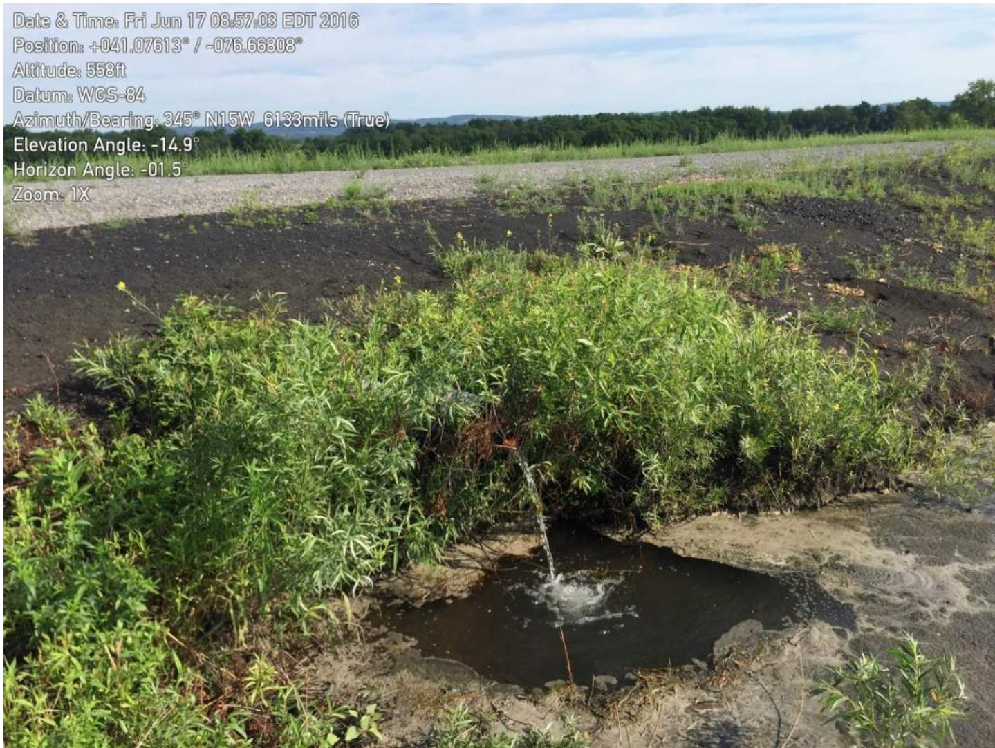
Photograph 10 – Seepage Collection System Outlet Pipe
