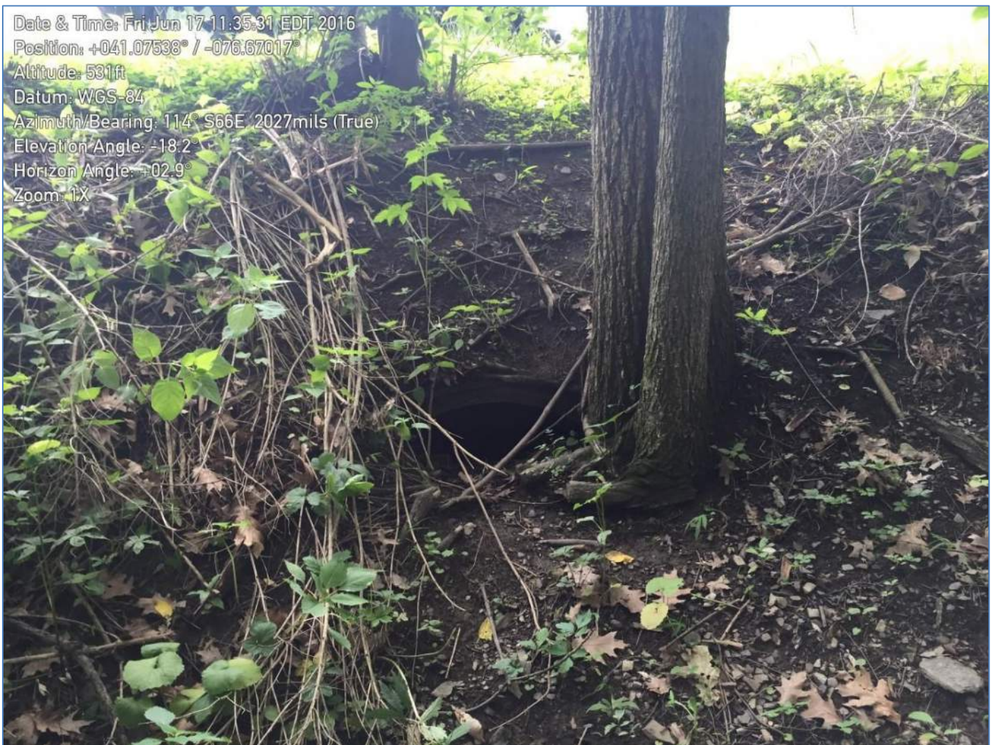
Photograph 9 –Abandoned Overflow Culvert Pipe Outlet (plugged)
