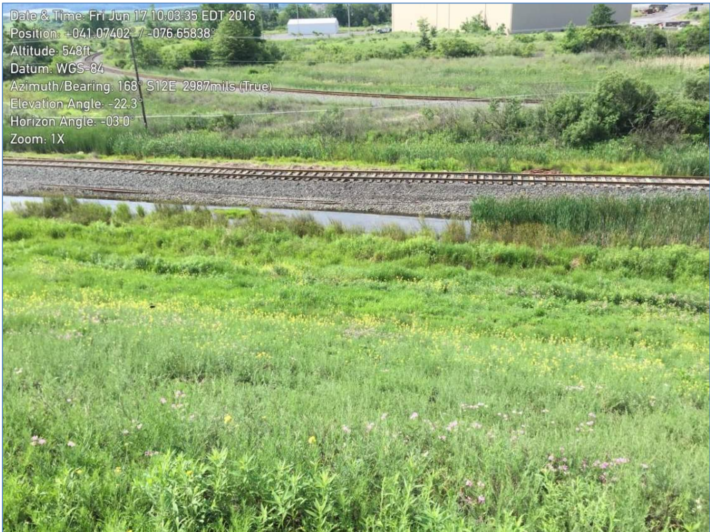
Photograph 4 – Ponding Water at Toe of Southwestern Dike Slope
